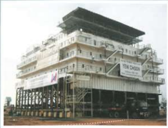
Shifting and ro-ro of Accommodation Module. Dim. 51.5m x 32.67m x 19.6m (1,400 Tons).
