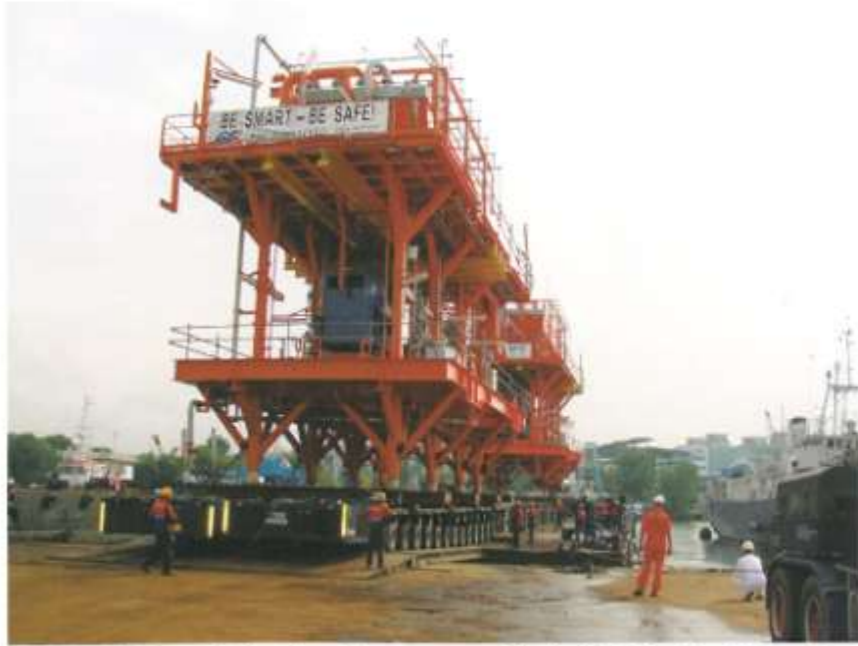
2 units HP Post Dehy Gas Compressor Module being loaded onto barge via ro-ro operation. Dim. 22m x 8.7m x 13.5m (375 Tons) each.
