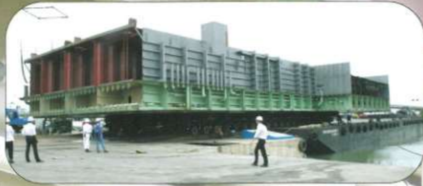
Singapore Load out of 700T Heavylift, 44.3 x 27 x 5m from fabrication yard to PPL Shipyard.
