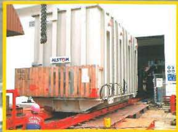
The skidding method is used to position this Transformer in an enclosed area.
